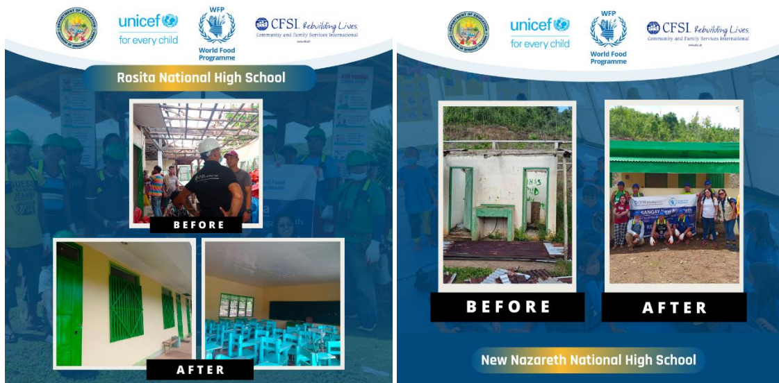
Before and After Photos of School Rehabilitations in the Schools Division Office of Dinagat Islands.
